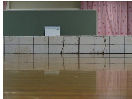
(b) The close-range image with clear crack characteristics.
